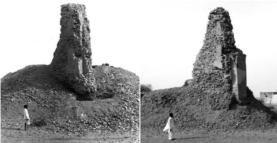
Figure 4. The Thul at Mansurah in 1897 (left from Cousens, 1929) and in 2008 (right). The integrity of this 12-m-high structure, which is bonded with a tough mortar, suggests that in the past millennium, the maximum shaking intensity in the region cannot have much exceeded Mercalli intensity X. The faced re-entrant corner remains approximately vertical. Cousens excavated through the foundation of the Thul to virgin soils at a depth of 5 m below ground level. The 3-m-thick walls enclosed a 2.2 m central spiral staircase leading to a well within.
